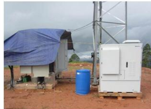
ElectraGen™ - ME backup power system installed at a base station in East Timor
